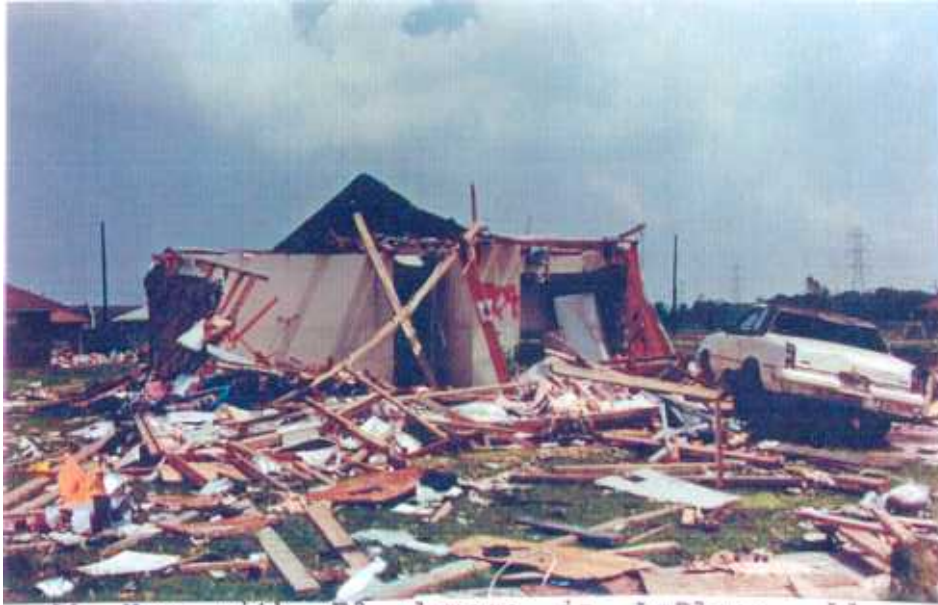
81. Home with F3 damage in LaPlace, LA tornado.
