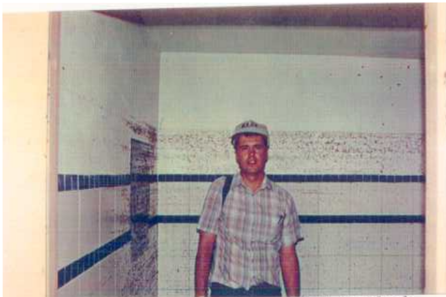
71. Water mark along restroom wall in Black Point Marina.
