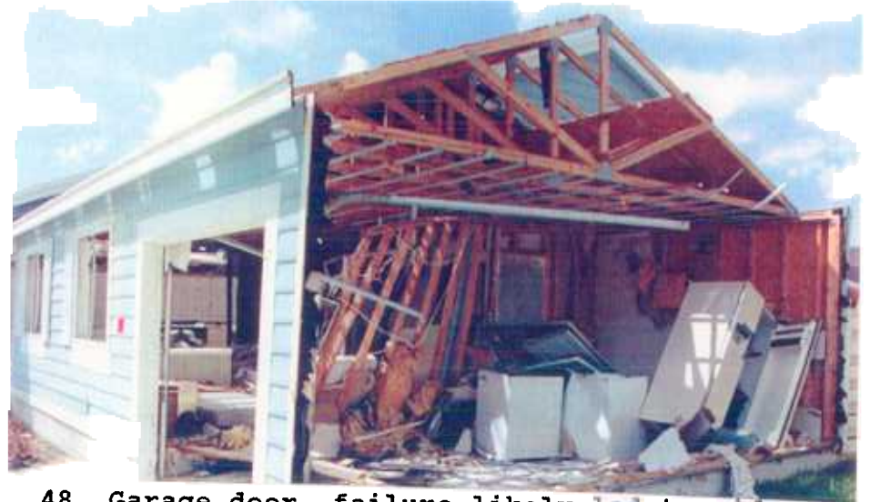
48. Garage door failure likely led to side wall collapse in Country Walk home. The door faced east; few nails secured the wall.
