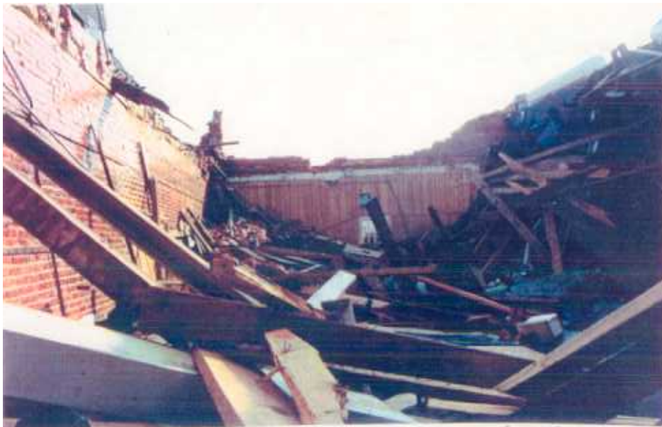
79. Timber roof collapsed in downtown Jeanerette, LA building.
