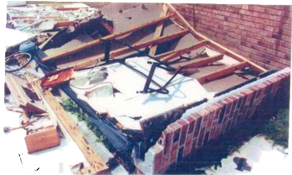
82. Exterior brick wall and framing rotated northward. Failure occurred where wall studs were nailed to anchored bottom plate.
