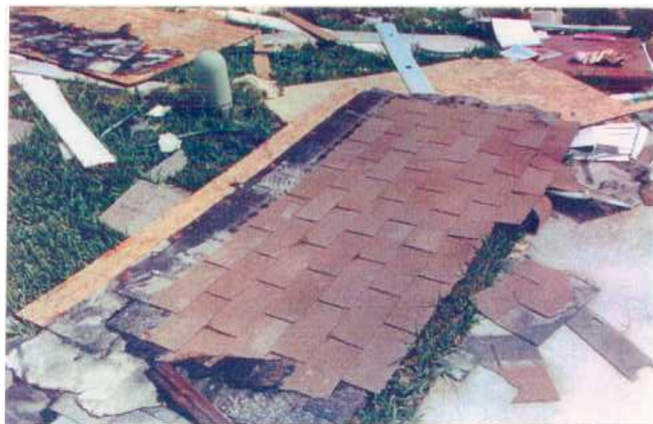
40. Full sheet of chipboard decking with shingles left intact (Homestead).
