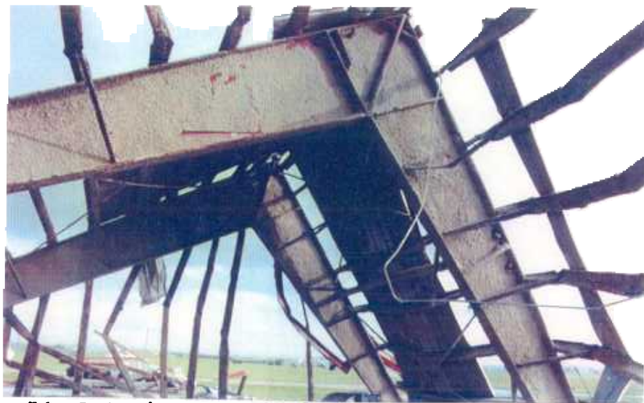
54. Rotation of steel frame occurred when center of hanger collapsed. View looking north at Tamiami Airport.
