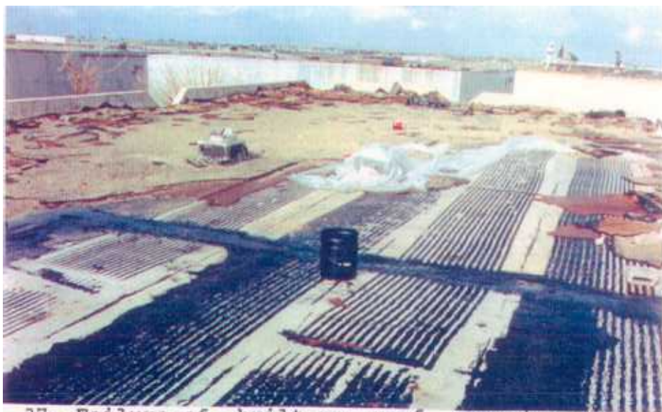
37. Failure of built-up roof covering on warehouse occurred where insulation board was lightly adhered to roof deck.
