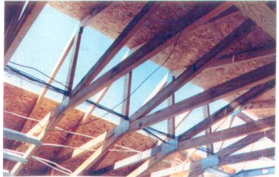
42. Lack of blocking between rafters in Homestead residence.
