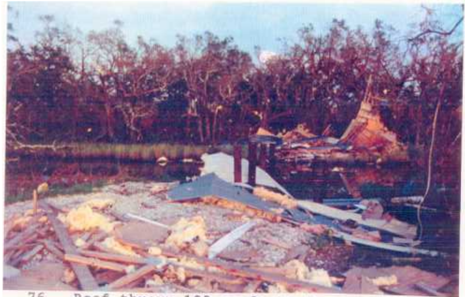
76. Roof thrown 100 yards to the south of residence depicted in previous photograph.
