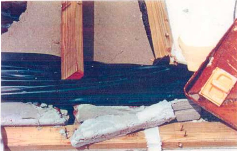
83. Wall studs were end nailed and were easily pulled from the bottom plate.
