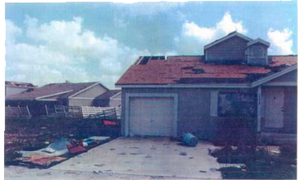
34. Roof shingles were stapled on house to the right and nailed on the house to the left (Country Walk).
