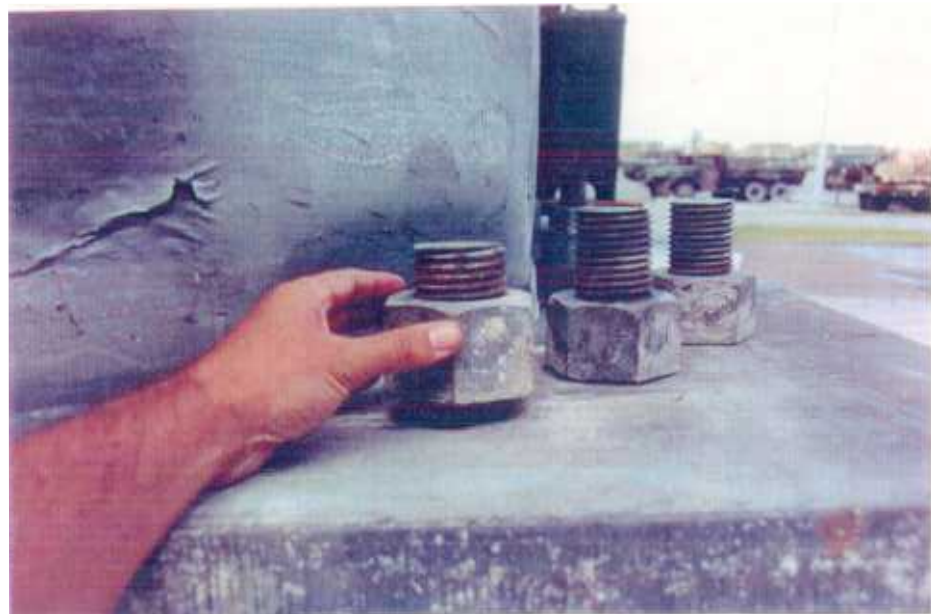
59. Nuts were loose on light standards base plate (Homestead).
