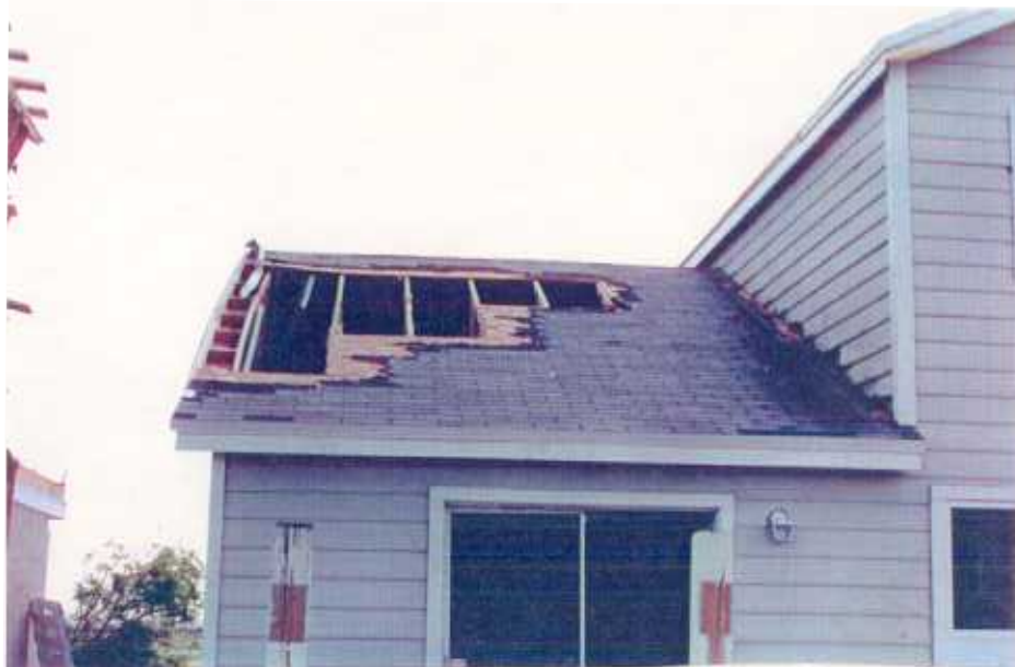
39. Missing full and half sheets of plywood decking on residence (Country Walk).
