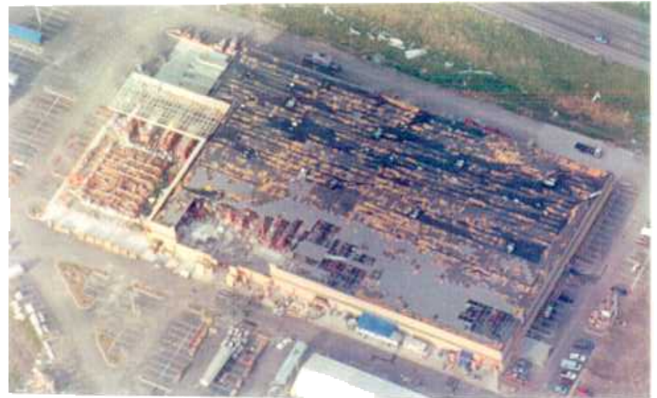
4. Loss of metal roof deck above department store entrance and northeast corner along Highway 1. View looking west.
