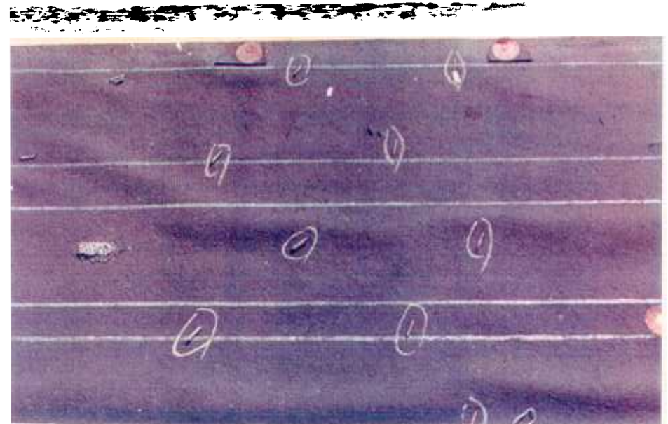
36. Staples oriented incorrectly on roof in Country Walk.
