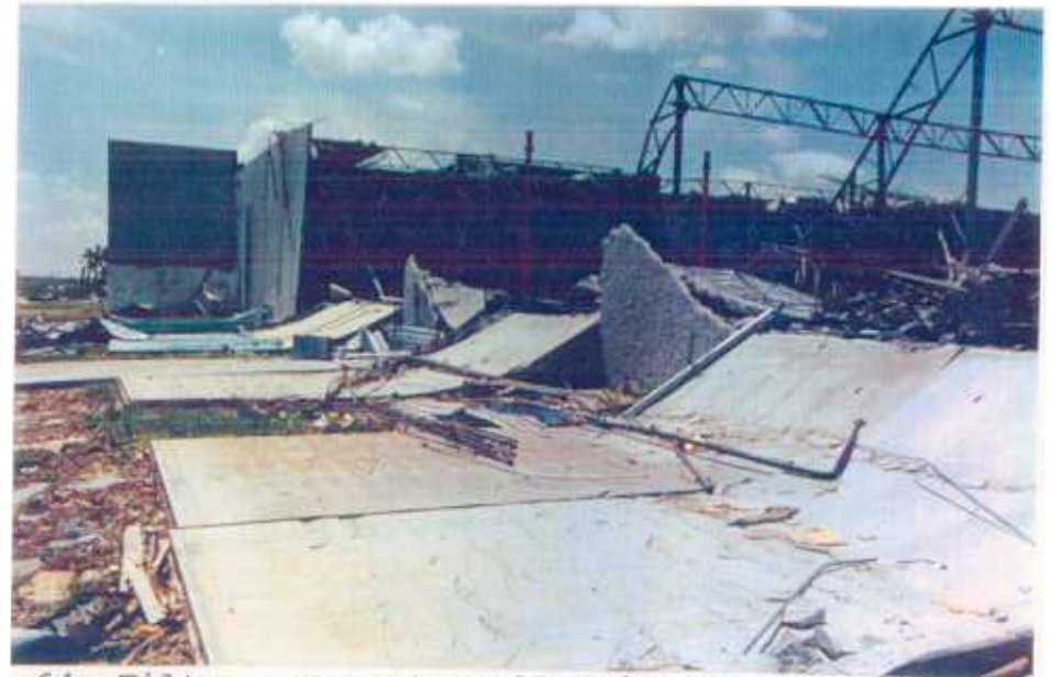
64. Tilt-up concrete wall failures on large warehouse. View looking southwest.
