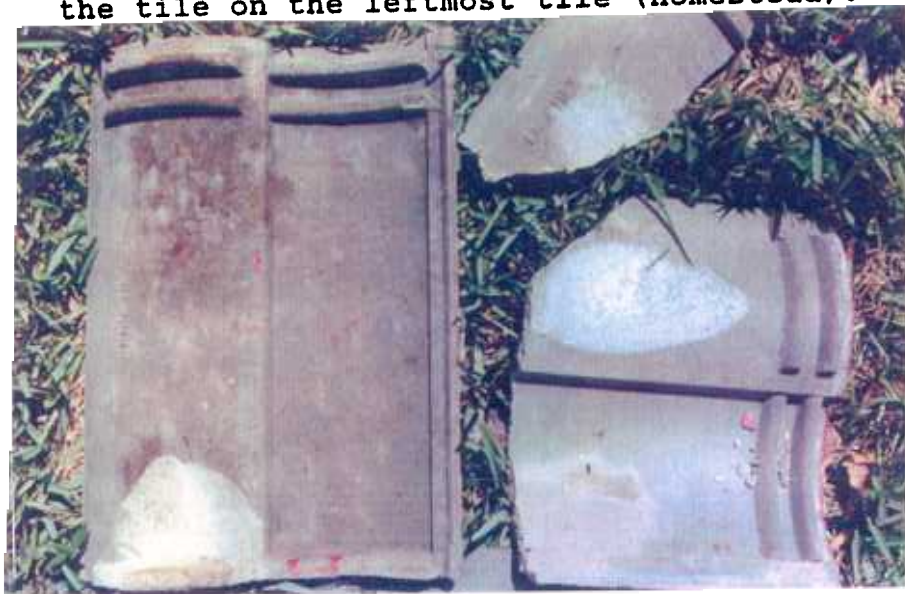
30. Tiles which did not bond well to mud. Note the offset between mud placement and the tile on the leftmost tile (Homestead).
