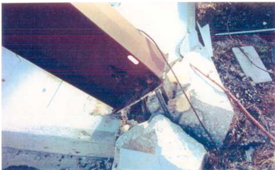
55. Rotation of column base caused steel bolts to pull loose from concrete footing. Note the base plate remained intact.
