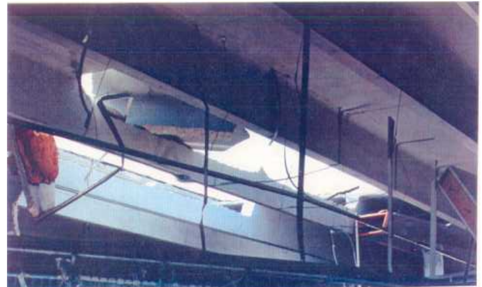
66. Unique failure of double-tee roof beam as it was uplifted in high winds on strip shopping center (Cutler Ridge).
