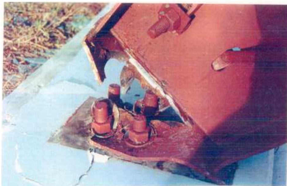
56. Torn base plate on airport hanger column (Tamiami Airport).
