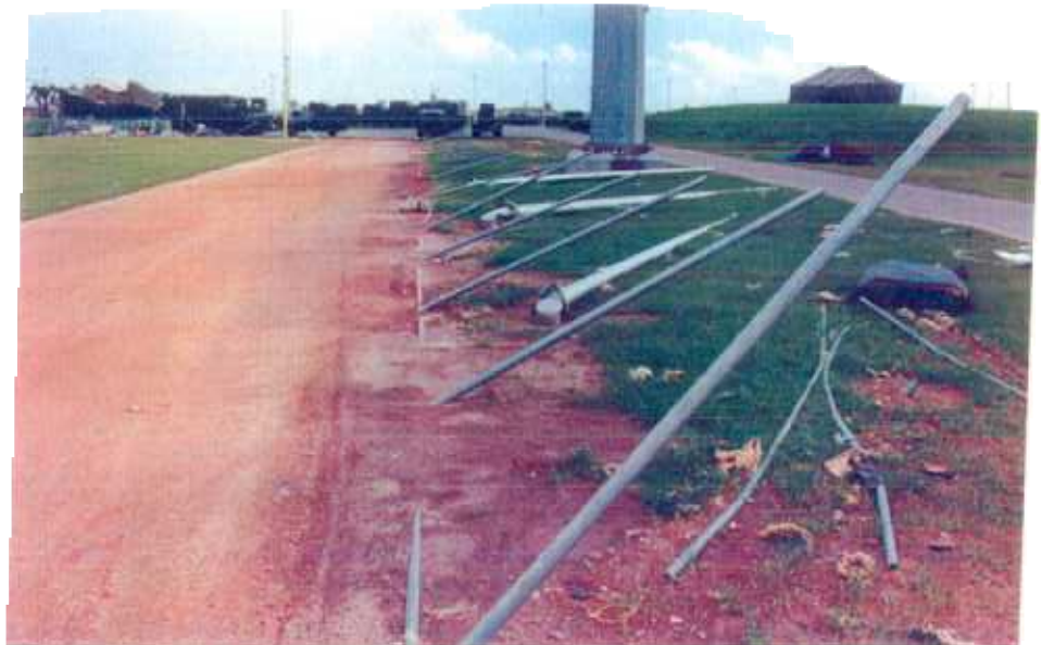
60. Fence along playing field downed to the east (Homestead)
