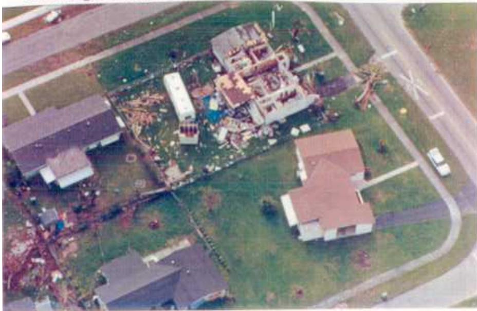
15. Loss of residence roof among undamaged homes. View looking southeast.
