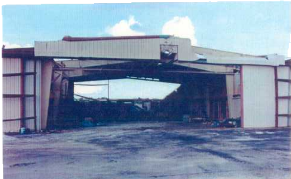
53. Hangar door and end wall failure in metal building at Tamiami Airport. Door faced east.
