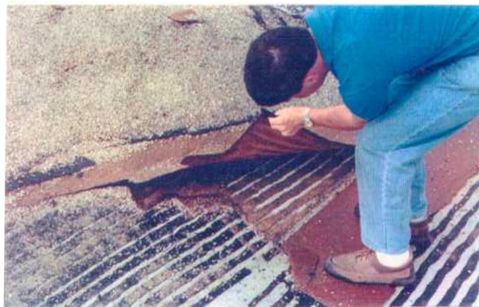
38. Insulation board had little to no bond to roof deck (near Tamiami Airport).
