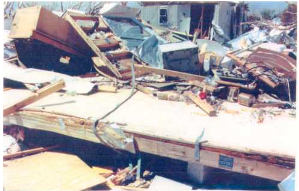
50. Mobile home steel frame and flooring are all that remained intact.
