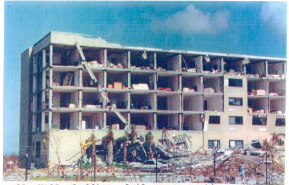
62. Wall cladding failure on suction side of condominium building along Saga Bay.
