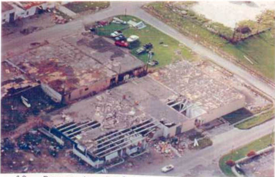
19. Damage to steel and concrete warehouse building in Florida City looking southeast.
