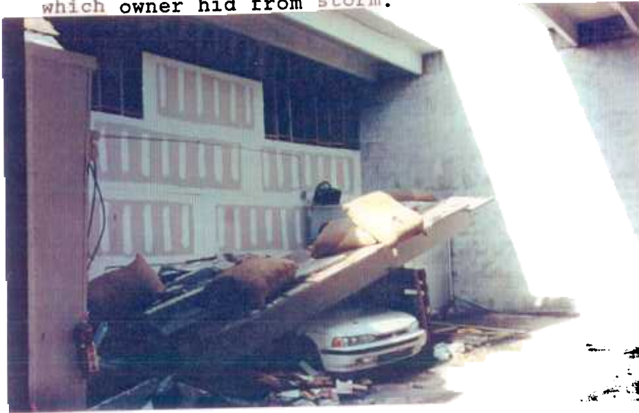
65. Double-tee concrete roof beam failed at center of 55 ft span and fell on top of car which owner hid from storm.
