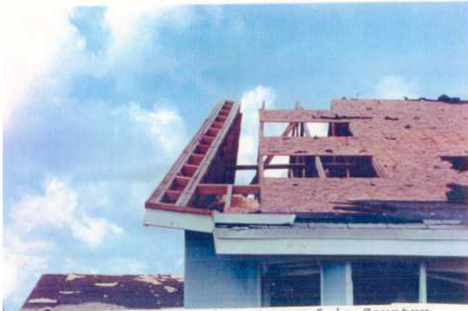
43. Gable end scabbed on to roof in Country Walk subdivision.
