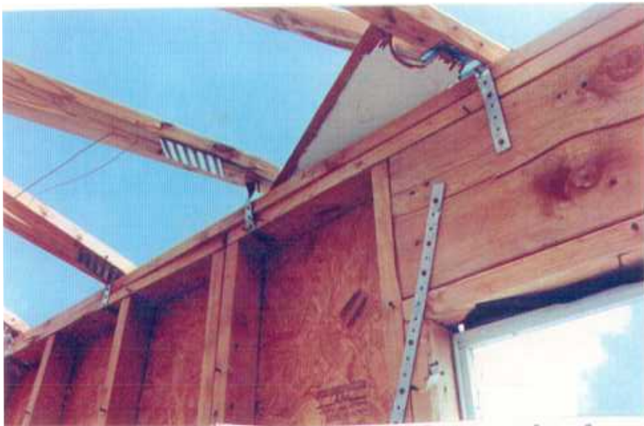
45. Rotation of metal straps along ends of roof trusses in residence.
