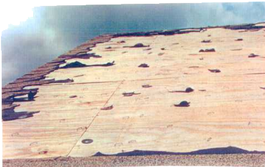
35. Close-up roof view showing staples secured in plywood deck. Many staples are crooked and oriented incorrectly.
