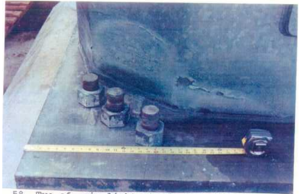
58. Two of six light standards had buckled slightly at base (Homestead).
