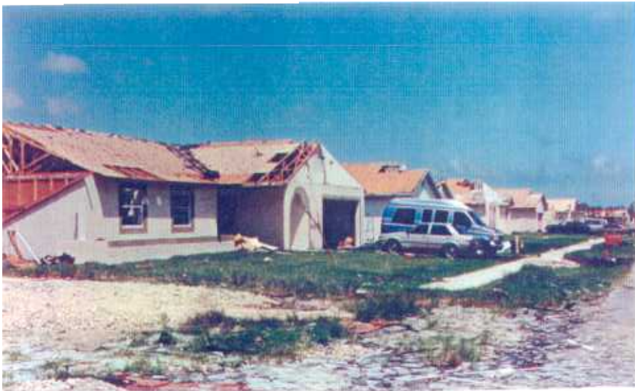
33. Almost complete absence of composition shingles on each house in subdivision just west of Homestead Air Force Base.
