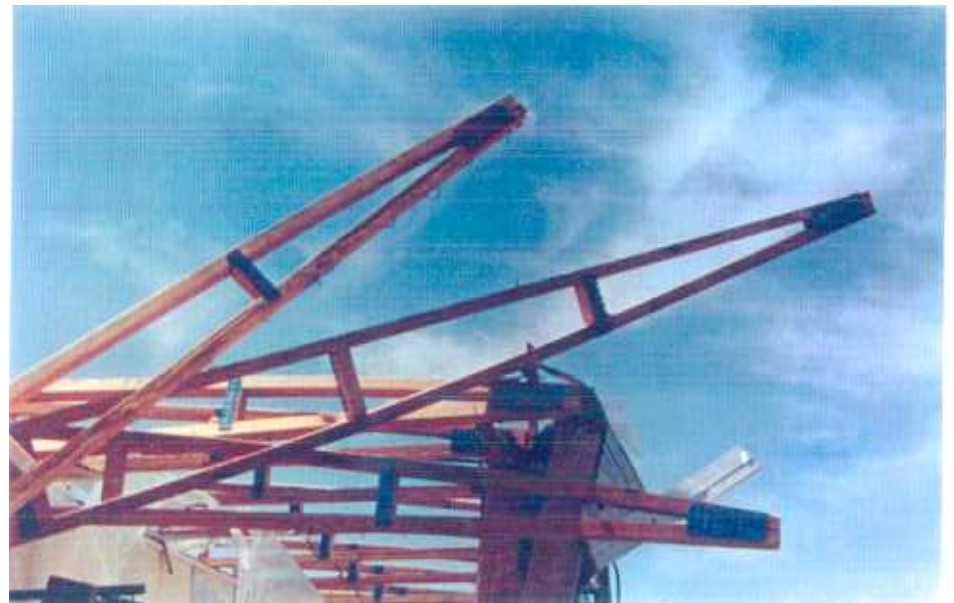
52. Roof trusses fell intact as they were lightly attached to the walls.
