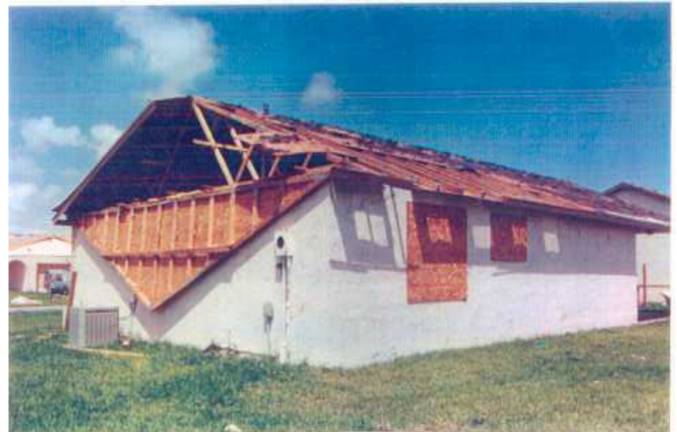
44. Gable end failures were common in several subdivisions in Homestead.
