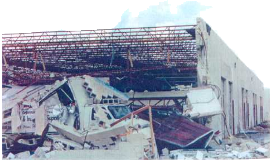
61. Northeast wall corner failure in concrete masonry warehouse near Tamiami Airport.
