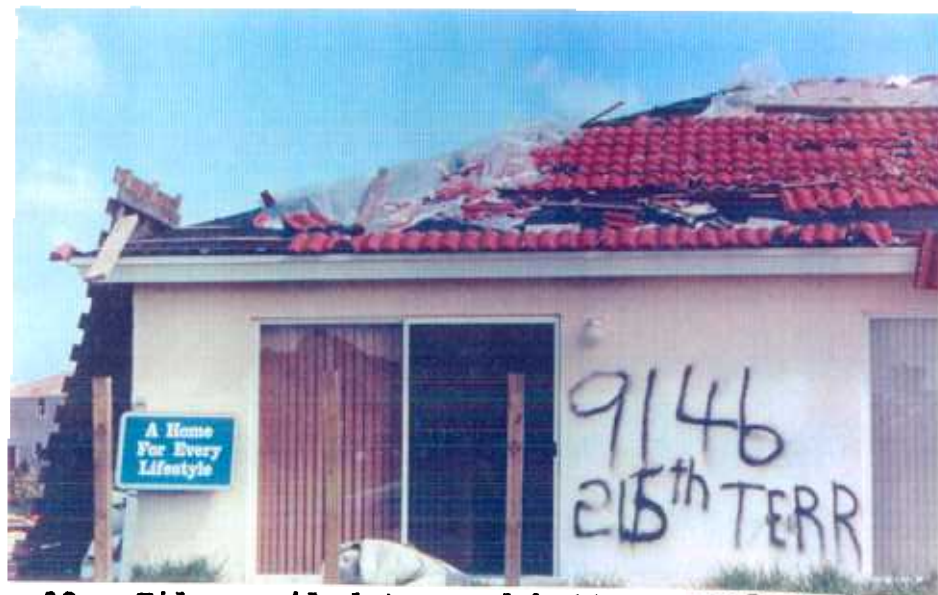
32. Tiles nailed to wood battens performed just as poorly as tiles that were mudded to roll roofing (Saga Bay area).
