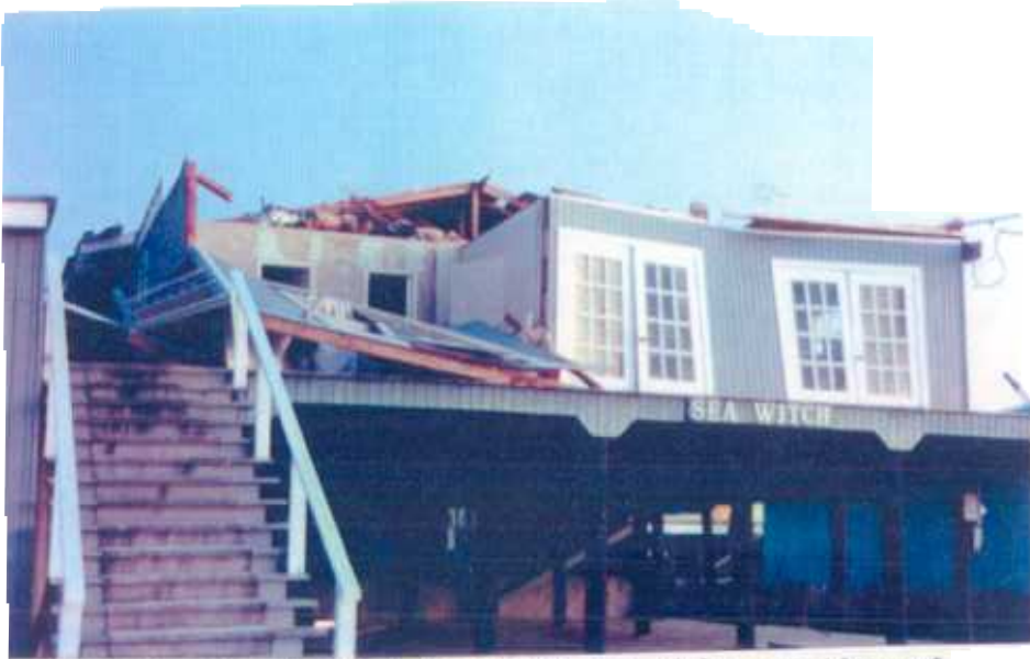
77. Windward wall buckled on this northward facing residence at Cypremort Point.
