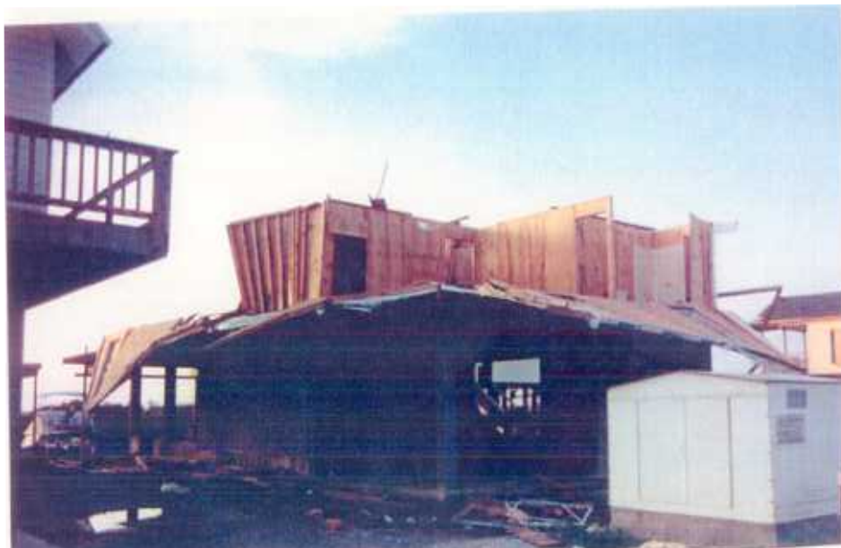
75. Loss of roof and exterior walls on residence at Cypremort Point, LA.
