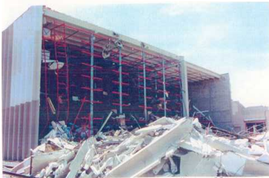
63. Large span double tee building collapse in Cutler Ridge. View looking southwest.
