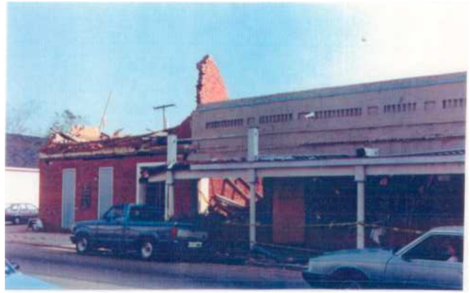
78. Collapse of old wood timber roof on main street in Jeanerette, LA.
