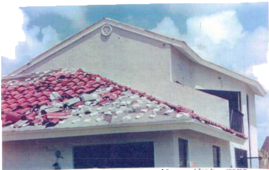
29. Damage to concrete tiles that were secured with mud (mortar). Failure occurred between the mud and the tile.
