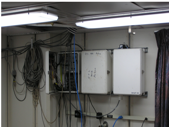
Data loggers in main computer room
