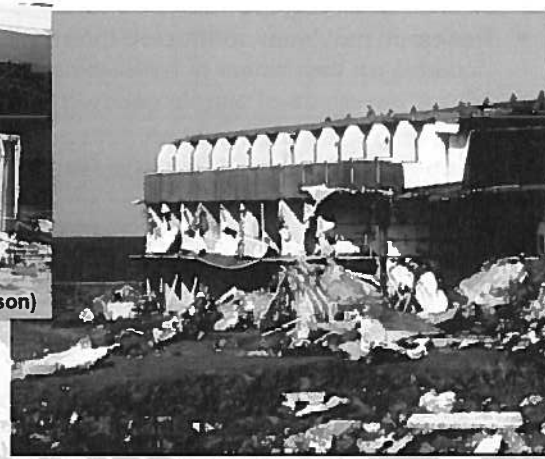
Hurricane Iwa, Poipu Village, Kauai, 1982 (Arthur Chiu) (Hotel was rebuilt at this site with same structural system just in time to be destroyed again in Hurricane Iniki 1992)
