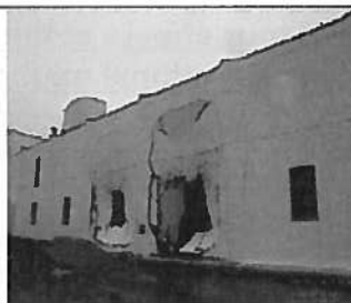
Minami Gamou STP Building 2011 (Lyle Carden) Video
