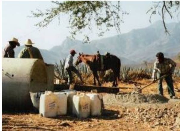
Photo G.16: Local people building a well to save river water in the SMBR
